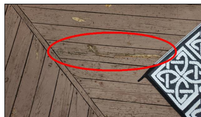
2.1 Item 4(Picture) Example/ Sample- deterioration/damage
