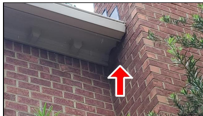
2.0 Item 4(Picture) Example/ Sample- left side of home – appears to be some deterioration
