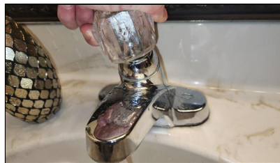
6.4 Item 5(Picture) Example/ Sample- Primary Bathroom Left Sink- water control handle leaks while operated, water control handle loose
