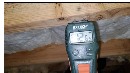
5.0 Item 3(Picture) Example/ Sample- front and rear of main house – Considered acceptable at time of inspection – wood moisture content(WMC) 12.6% +/-
