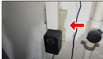
7.5 Item 2(Picture) Example/ Sample- Garage- cover damaged, loose outlet
