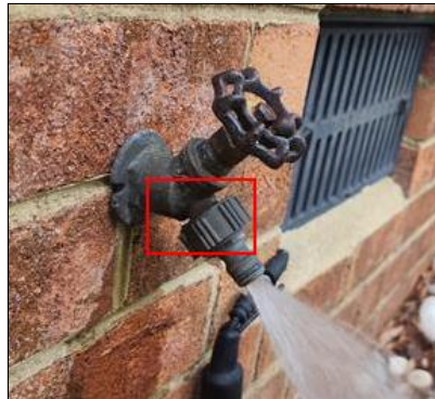
6.4 Item 2(Picture) Example/ Sample- Left side of Home, Rear of Home- leaks while in use (this waste water)
