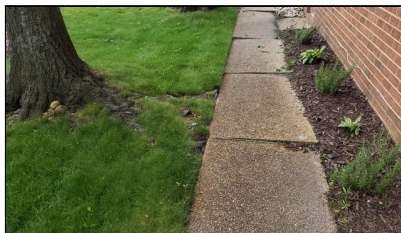
2.2 Item 7(Picture) Example/ Sample- left side of home sidewalk – trip hazards
