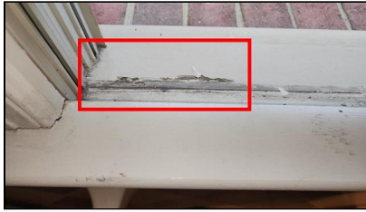
2.0 Item 10(Picture) Example/ Sample- Rear of home- deterioration
