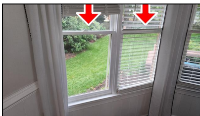
3.5 Item 2(Picture) Example/ Sample- Sunroom- Stuck shut
