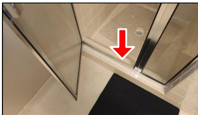
6.4 Item 4(Picture) Example/ Sample- Primary Bathroom Shower door has to be lift up to close and open
