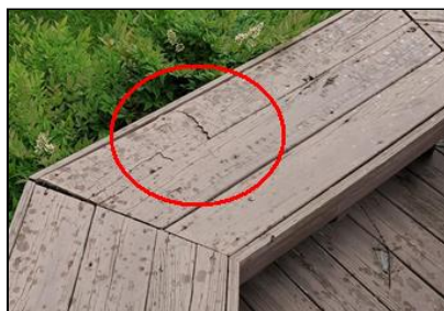
2.1 Item 3(Picture) Example/ Sample- deterioration/damage
