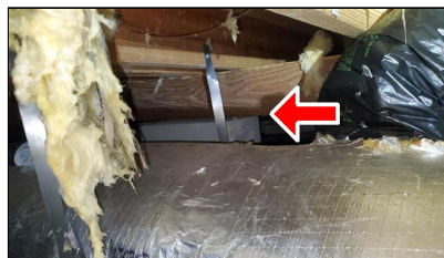
5.0 Item 2(Picture) Example/ Sample- rear of home near the right side –beam not resting on Piers properly – possibly just needs shims
