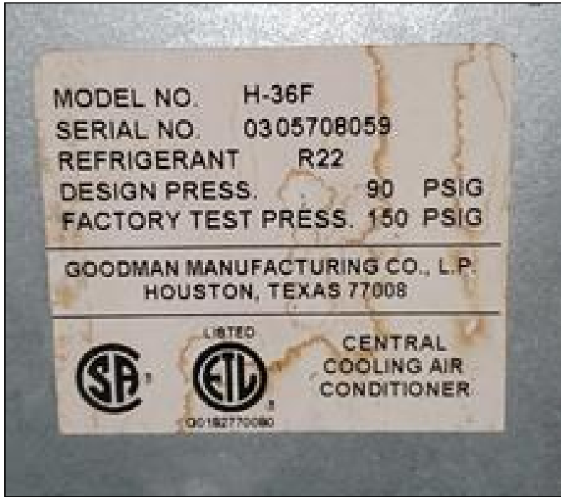
AC coil label – located in the attic – GOODMAN MANUFACTURING – manufacture year 2003
