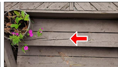
2.1 Item 2(Picture) Example/ Sample- deterioration/damage
