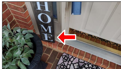
2.0 Item 5(Picture) Example/ Sample- rusted components such as front sidelite
