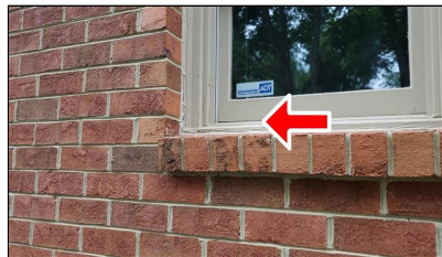
2.0 Item 2(Picture) Example/ Sample- rear of home – deterioration
