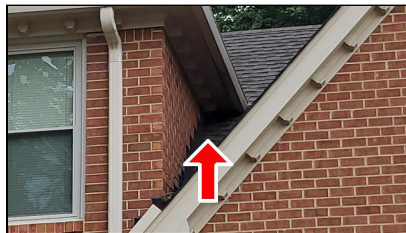
2.0 Item 1(Picture) Example/ Sample- Front of home- paint finish deficiency
