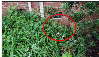
8.5 Item 2(Picture) left side of home – Appears to be a condensation drain line
