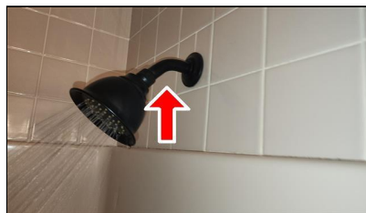
6.4 Item 8(Picture) Example/ Sample- Second level Hall Bathroom Shower- shower supply pipe is loose
