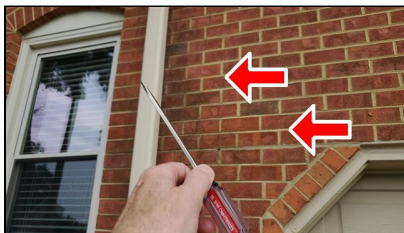
2.0 Item 11(Picture) Example/ Sample- front of home cracking
