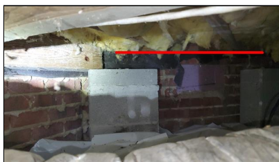
5.0 Item 8(Picture) Example/ Sample- floor joist not supported at end properly – appears that beams or missing observed at the addition area at the rear
