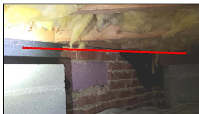
5.0 Item 7(Picture) Example/ Sample- floor joist not supported at end properly – appears that beams or missing observed at the addition area at the rear
