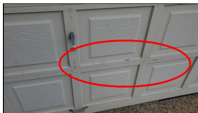
2.0 Item 7(Picture) Example/ Sample- front of home – garage – paint finish deficiency
