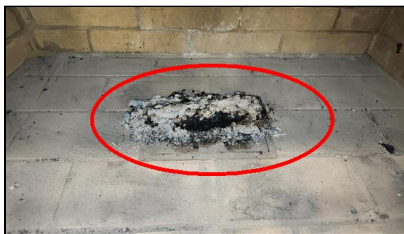
8.7 Item 1(Picture) Example/ Sample- ash buildup
