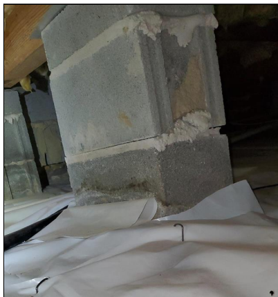
5.0 Item 5(Picture) Example/ Sample- masonry pier missing mortar slight movement possibly – consider sealing and monitor
