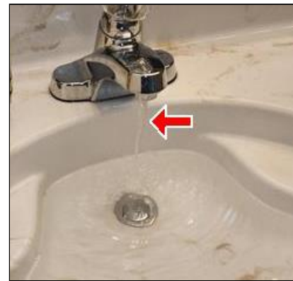
6.4 Item 6(Picture) Primary Bathroom Left Sink- The water pressure was reduced
