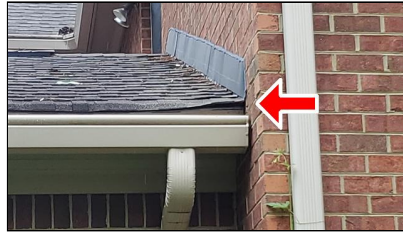
1.0 Item 2(Picture) Example/ Sample- left side of home – exposed sheathing, lifted risen shingle
