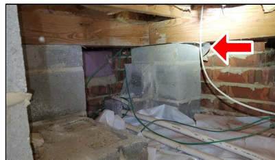
5.0 Item 6(Picture) Example/ Sample- left side of home – addition area beam not resting on pier properly
