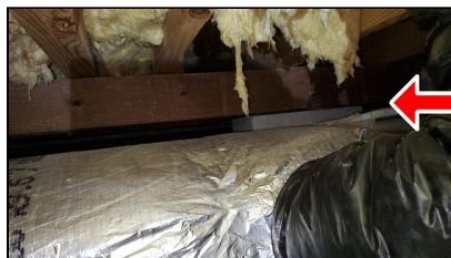
5.0 Item 1(Picture) Example/ Sample- rear of home near the right side –beam not resting on Piers properly – possibly just needs shims
