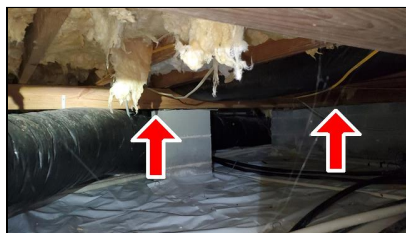
7.4 Item 1(Picture) Example/ Sample- loose wires
