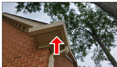
2.0 Item 8(Picture) Example/ Sample- front of home – possible deterioration
