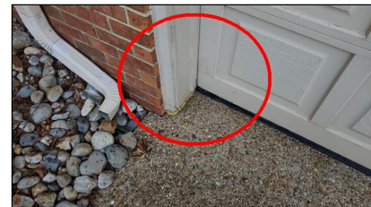
2.0 Item 6(Picture) Example/ Sample- front of home – paint finish deficiency
