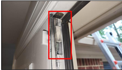
3.2 Item 1(Picture) Example/ Sample- Rear Door does not unlock
