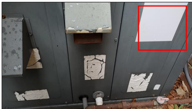
HVAC packaged unit label – located at the rear of the home – GOODMAN MANUFACTURING – manufacture year unknown labeling faded not readable – appears aged
