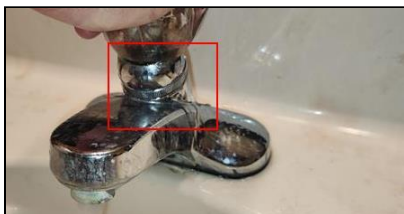
6.4 Item 7(Picture) Example/ Sample- Second level Hall Bathroom Sink- water control handle leaks while operated
